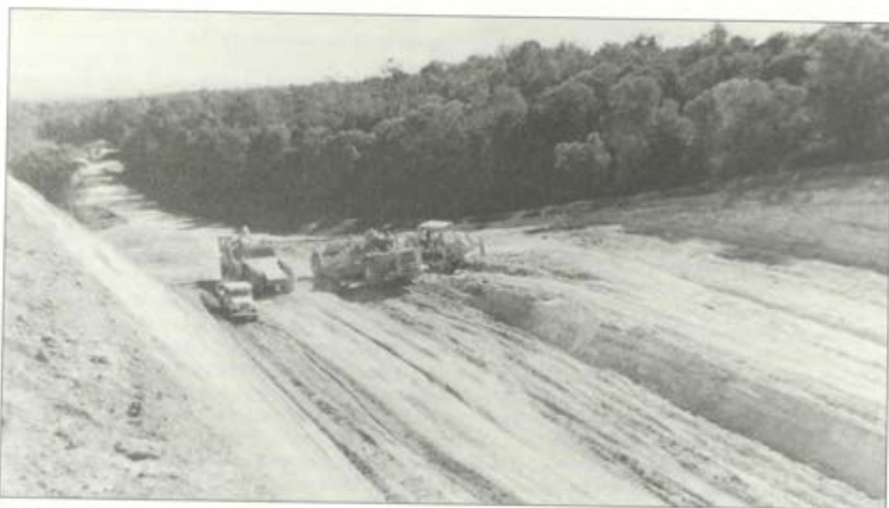
Rocky Creek access road, part of the extensive earthworks undertaken by the contractor — Thiess Bros. 6 June, 1980.
