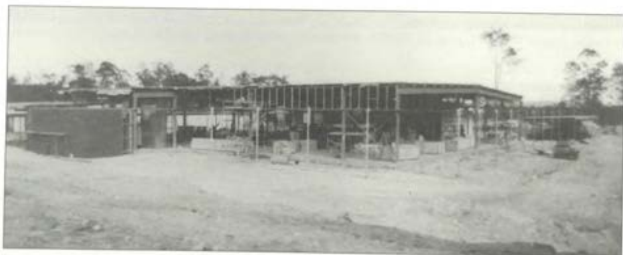
New construction office, showing No 1 plant room and condenser for air conditioning, constructed by R.F. James Pty. Ltd. 1 July, 1980.
