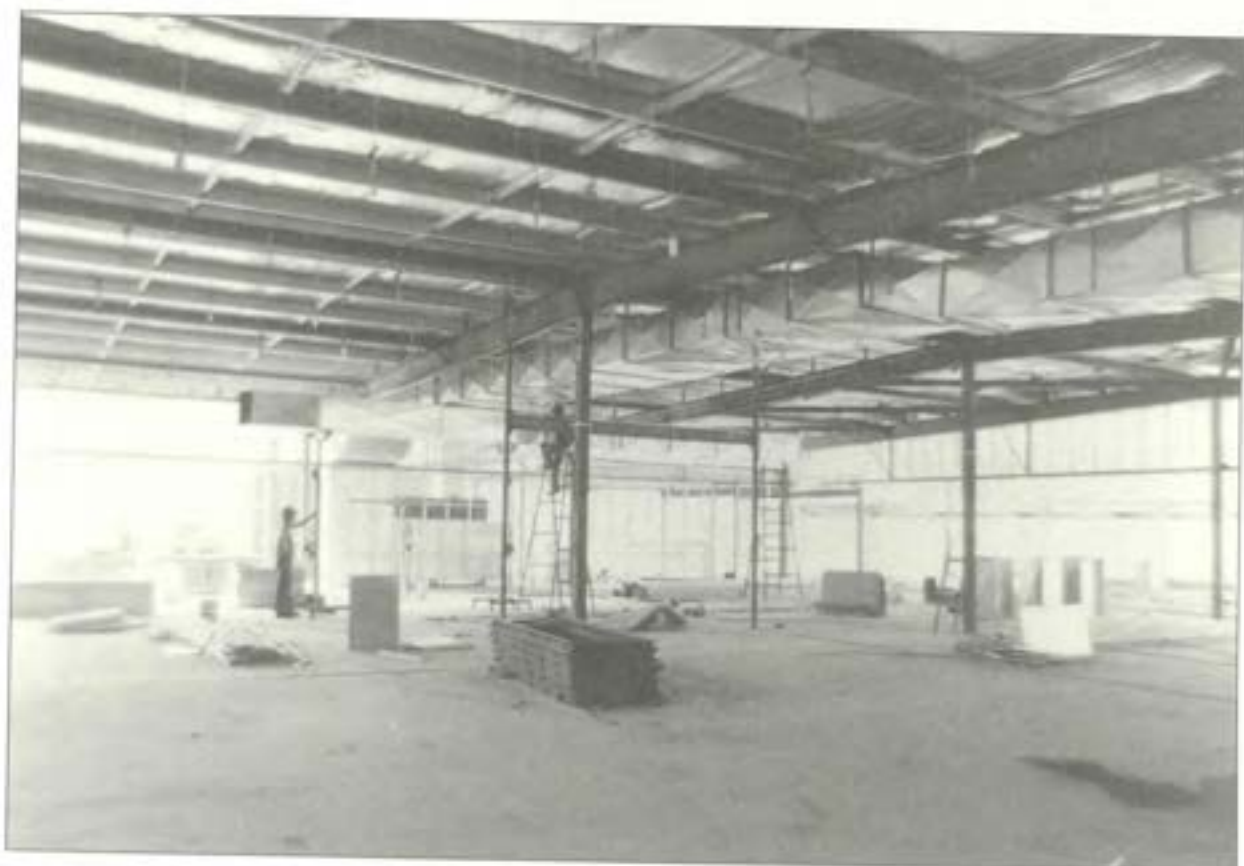
Interior view of the new construction office, showing air conditioning ducts and hangers prior to installation of frames to support the suspended ceiling. 1 July 1980.
