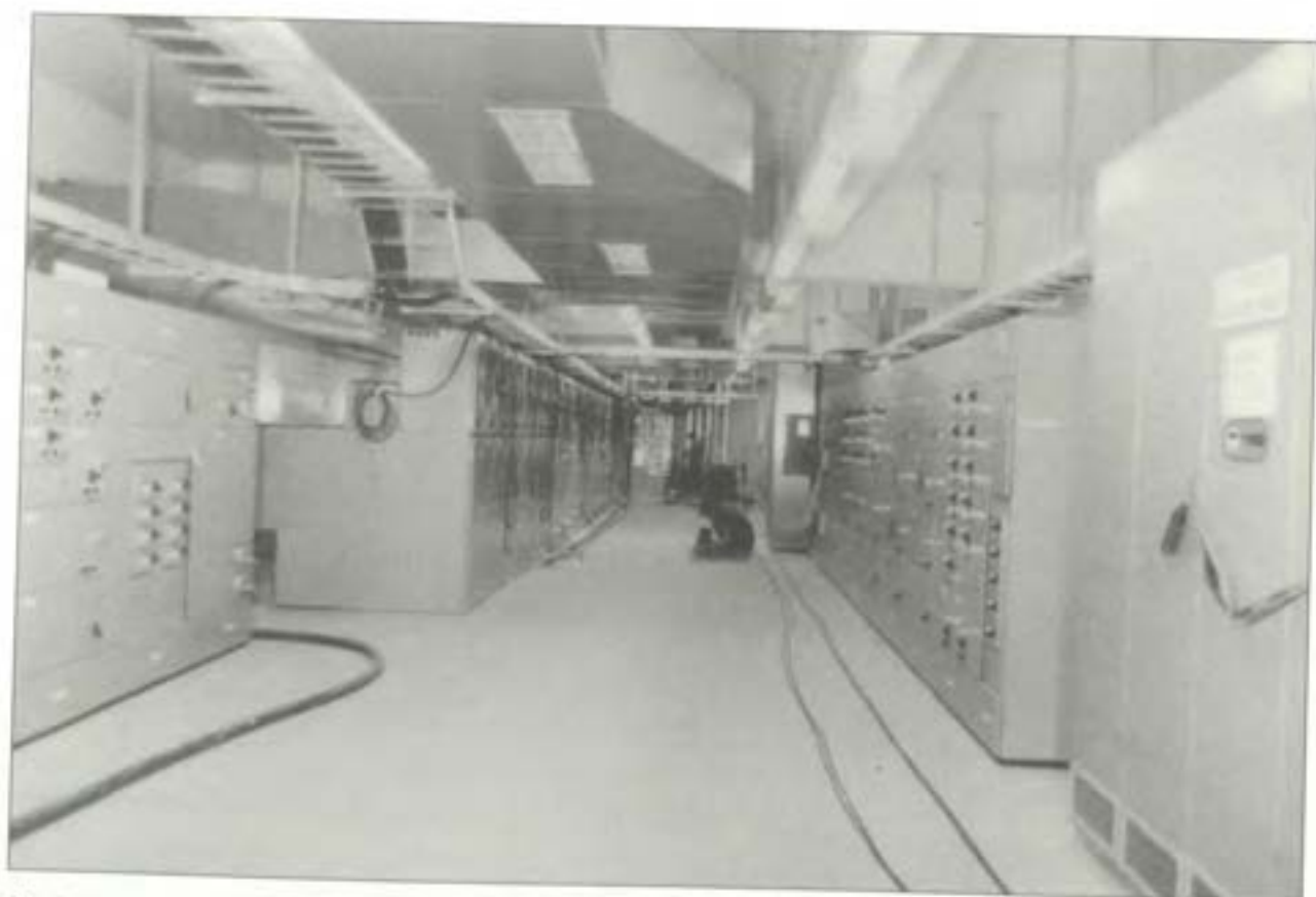
No 2 unit 6.6kV switchgear (Hawker Siddeley, left rear). 415V switchgear (G.E.C. — foreground). 2 February, 1984.
