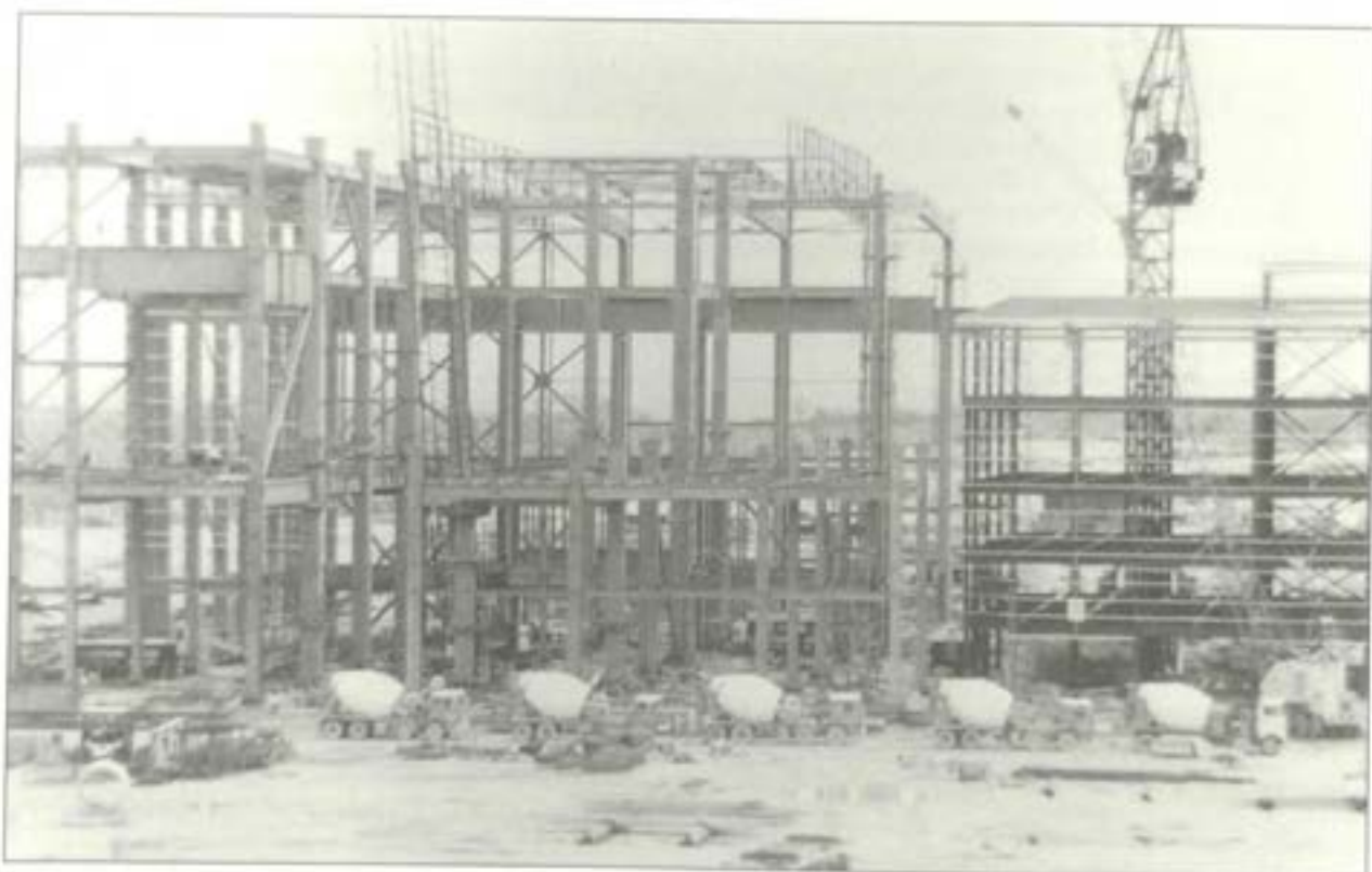
This view shows the progress of No 1 boiler house, rows 5, 7 and 9 of the turbine house and purlins and girts affixed to the No 1 annexe. Trucks are delivering concrete to the P.F. mills in No 2 boiler house. 7 April, 1981.
